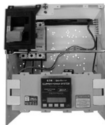
MCC Unit (Door Removed)
